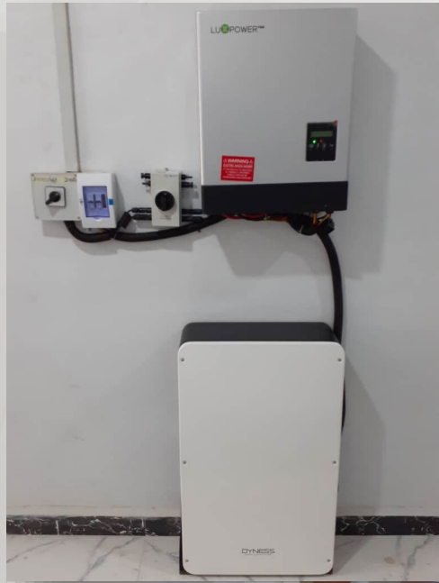
Address: Nigeria Capacity: 5kW/9.6kWh Function: Backup power
