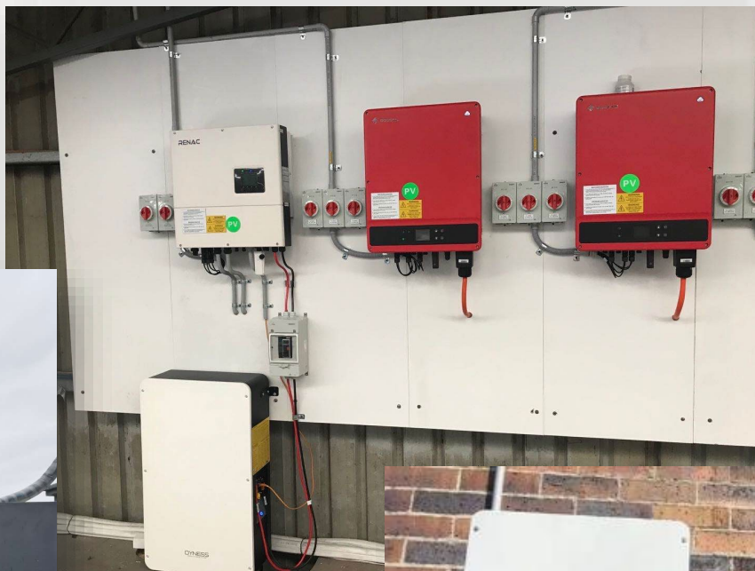
Address: Australia Capacity: 5kW/9.6kWh Function: Integrated renewable energy
