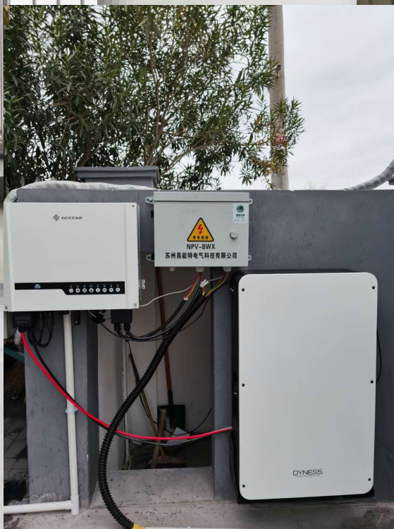
Address: Suzhou, Jiangsu Province Capacity: 5kW/9.6kWh Function: Backup power support
