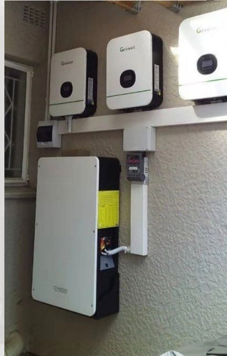
Address: Thailand Capacity: 3kW/9.6kWh Function: Backup power
